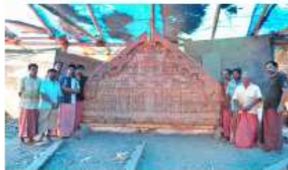
New Mukappa, after work with the craftsmen, it took 6 months to complete
