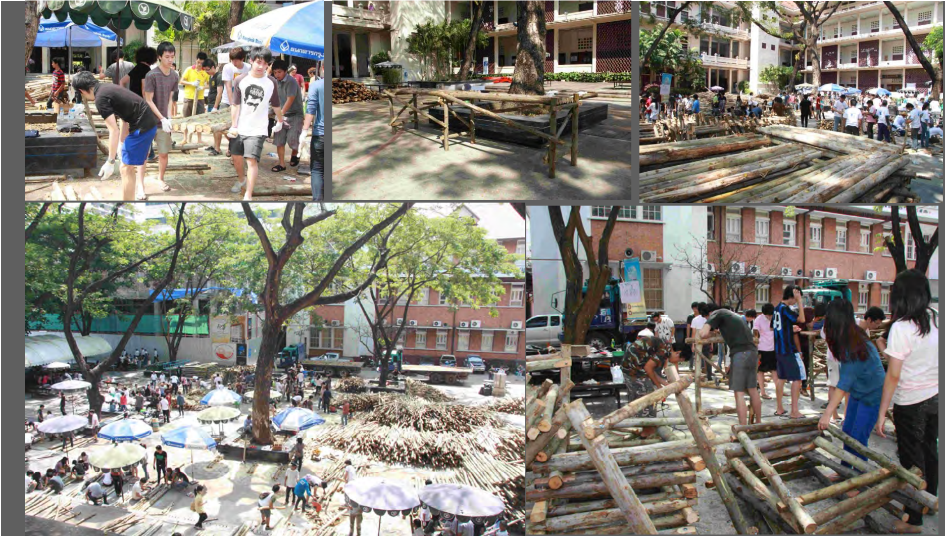
Chulalongkorn University students helping ASA and University to build temporary narrow board walk for the neighborhood to access to the main Public Transportation
