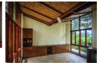
BAMBOO THATCH FALSE CEILING IS USED. WARM AIR PASSES THROUGH THE GAP IN THE MIDDLE OF TWO PARTS OF THE FALSE CEILING ENSURING LOW INDOOR TEMPS.
