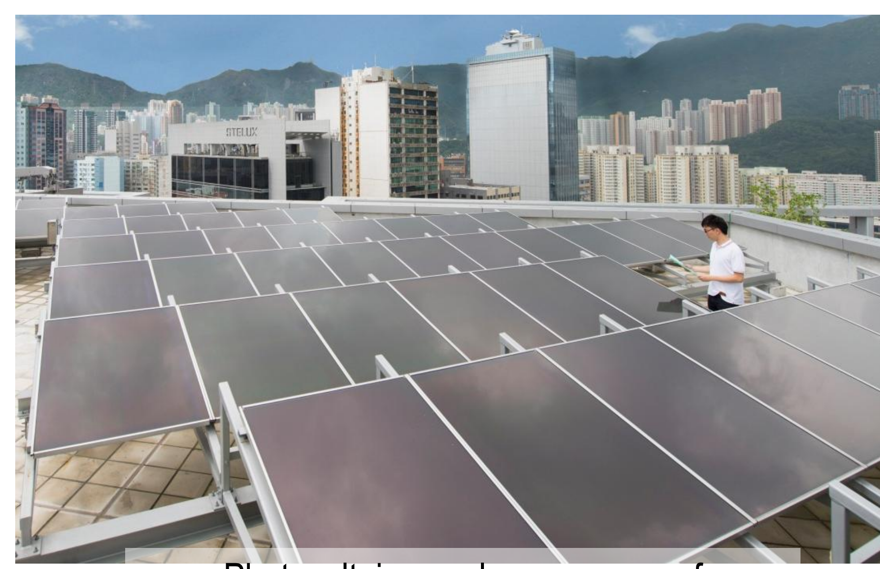
Photovoltaic panels on upper roof
